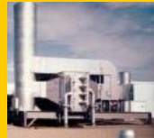
Heat recovery systems
