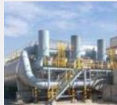
Solvent recovery systems
